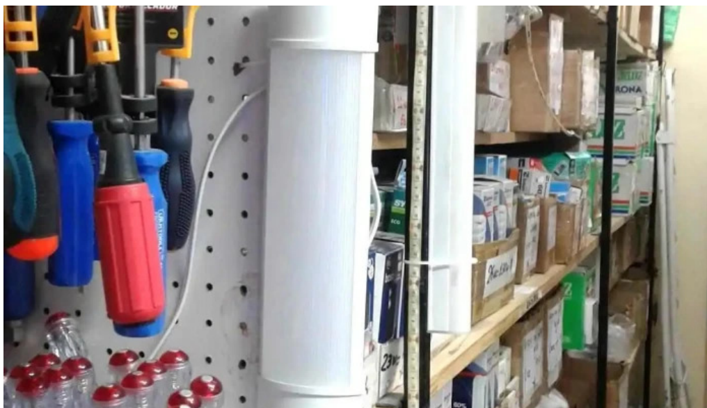
Mas luz electricidad interior
